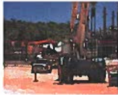
Contract personnel and heavy equipment can be seen as work continues along a roadway, just past the turnoff to the Guam National Wildlife Refuge, on March 31. The roadway is being installed near Ritidian Point to allow easier access to an area designated for several live-fire training ranges. RICK CRUZ/PDN
